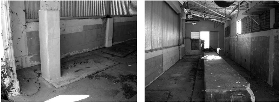
Figure 55. Optical alignment building 32 showing smaller pedestal with post (left) and larger pedestal (right) (ERDC-CERL 2007).
