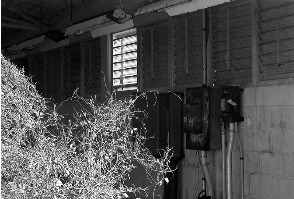
Figure 57. Interior of optical alignment building 31 showing louvered windows and electrical panels (ERDC-CERL 2007).
