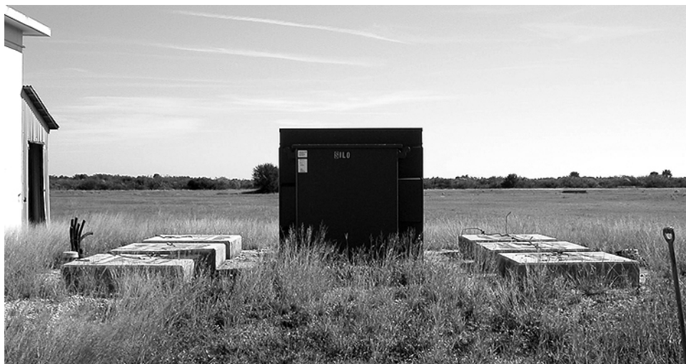
Figure 67. Launch support building transformer vault (ERDC-CERL 2007).
