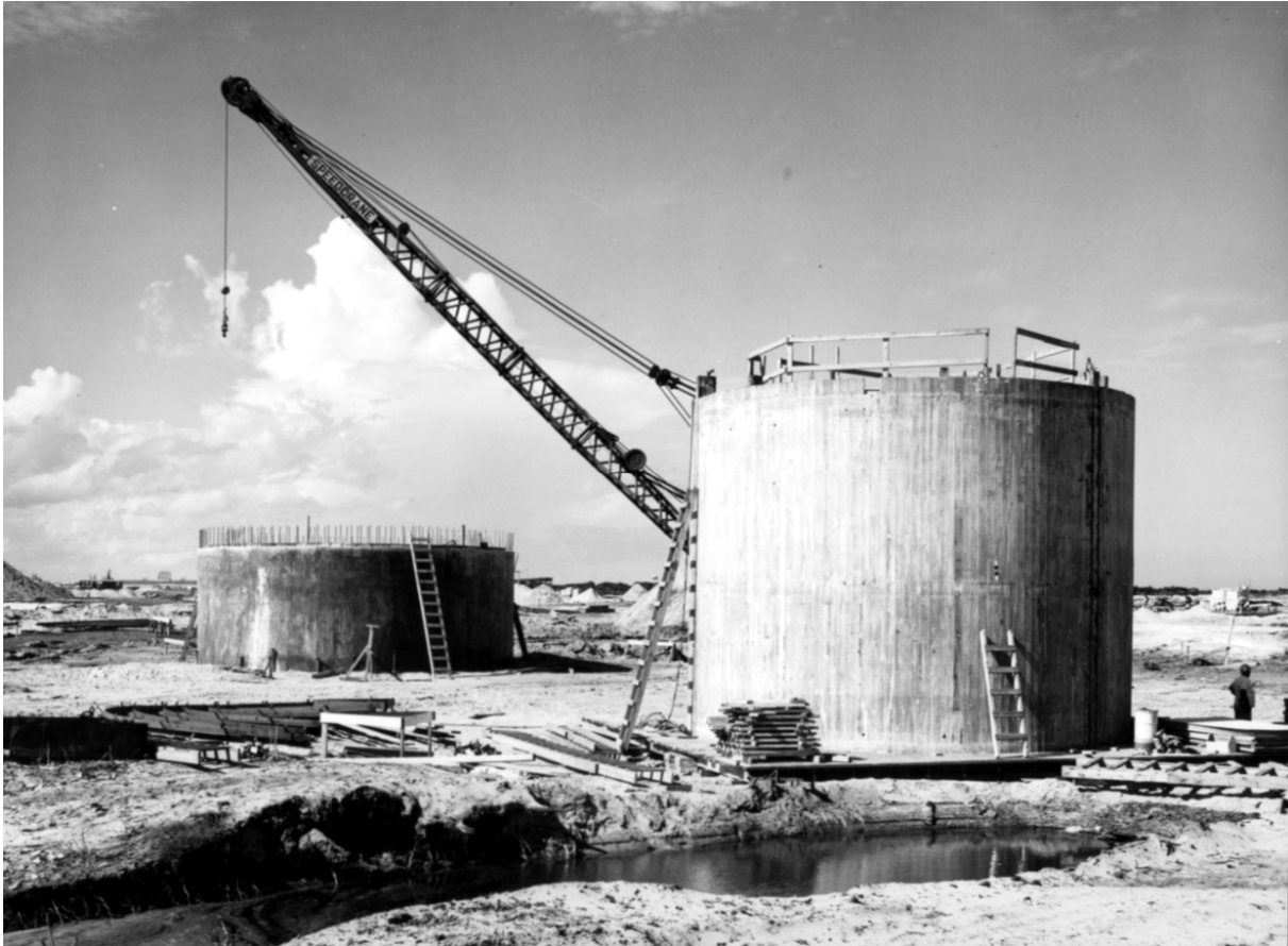
Figure 16. Construction of silo and R&D room, 30 October 1959 (NARA). Smaller concrete structure to the left may be the next ring to get stacked on the silo (right).
