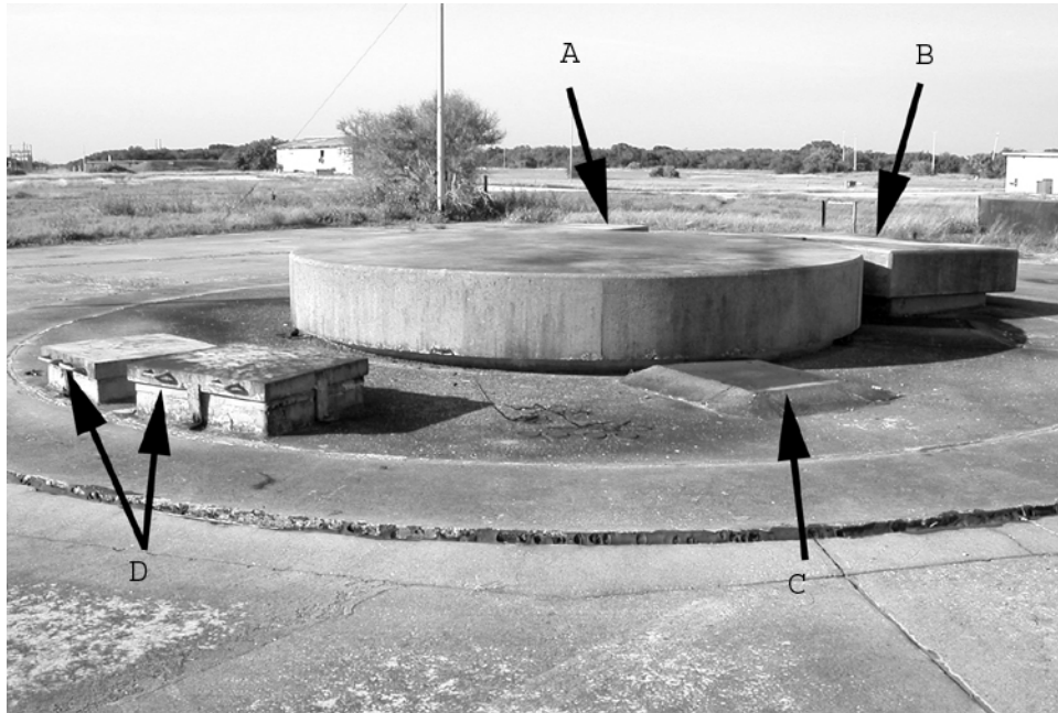
Figure 59. Silo 31B showing (A) guidance alignment notch, (B) personnel and equipment access hatch, (C) T-E jack point, and (D) junction-box openings (ERDC-CERL 2007).
