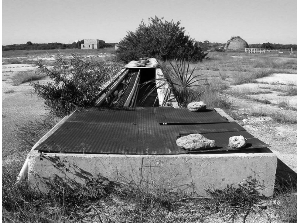
Figure 73. Cableway transition II near pad 31 equipment room (ERDC-CERL 2007).
