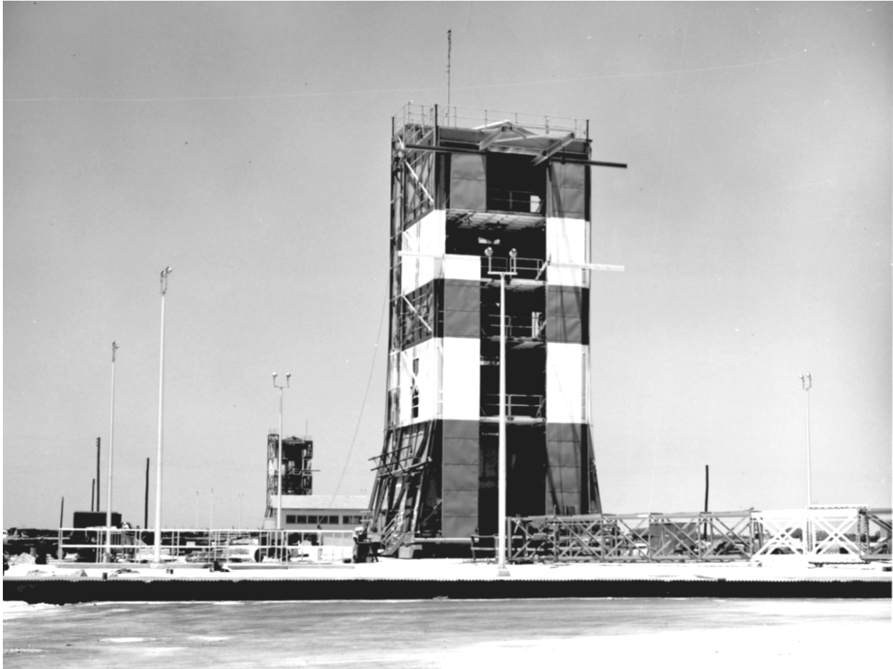
Figure 18. Completed mobile service tower for pad 31A, 29 July 1960 (NARA). The tower for pad 32A is visible in the background with an optical alignment building in between.
