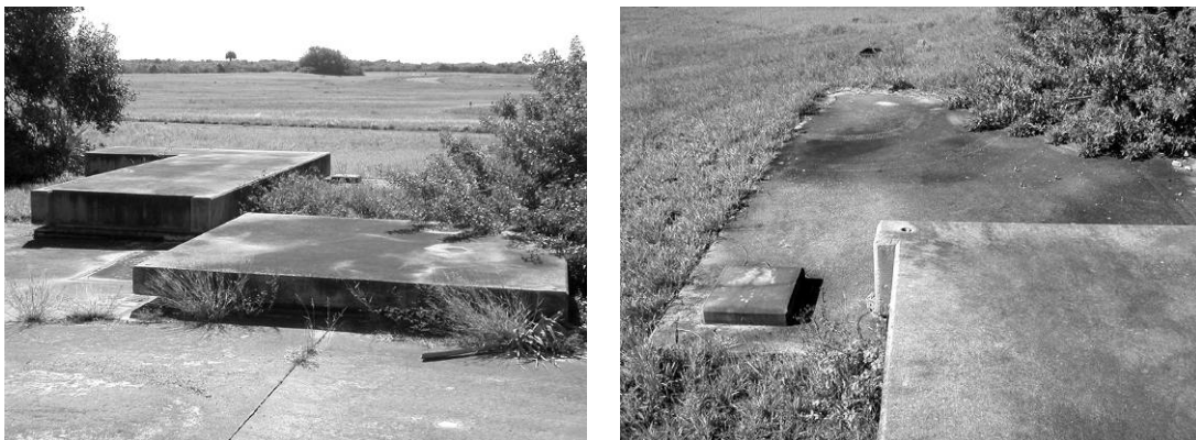
Figure 60. Removable concrete covers over Silo 32B R&D equipment room (left foreground) and subterranean staircase (left background; right foreground); concrete roof with corner exhaust vent of transformer vault (right background) (ERDC-CERL 2007).
