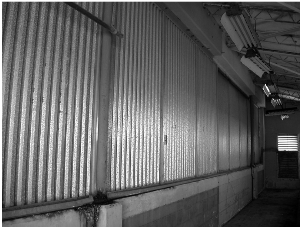
Figure 54. Sliding doors in optical alignment building 32 (ERDC-CERL 2007).
