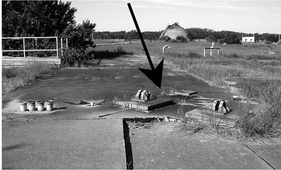
Figure 48. Pad 32 pad equipment room umbilical tower mounting (ERDC-CERL 2007).
